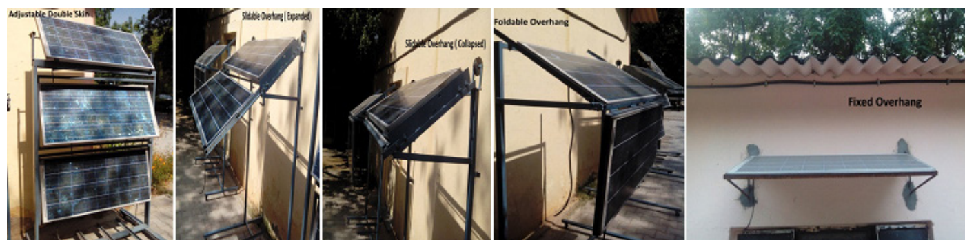
Figure 20: BIPV prototype developed and being monitored
